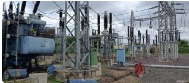
Substation augmentation at Shendra, Aurangabad, MH | 220 kV
