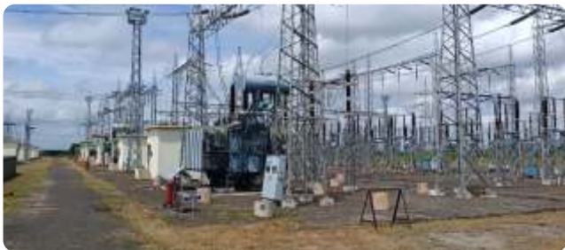
Substation Augmentation at Chikalthana, Aurangabad, MH | 132 kV
