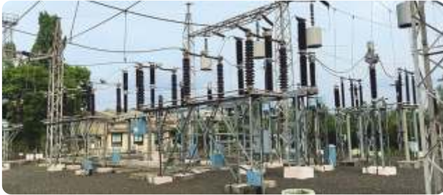
Substation Augmentation at Talegaon, Wardha, MH | 132kV
