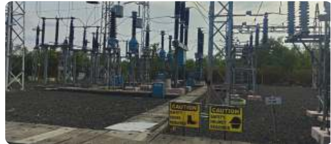
Substation augmentation at Saoner, Nagpur, MH | 132 kV
