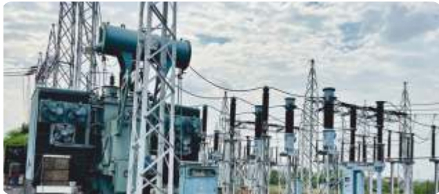
Substation Augmentation at Kanhan, Nagpur, MH | 132 kV
