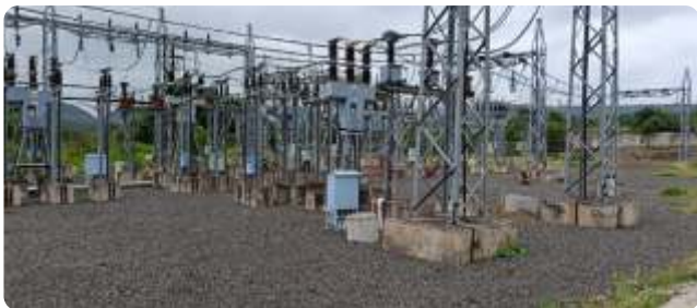
Substation Augmentation at Amgaon, Gondia, MH | 132kV
