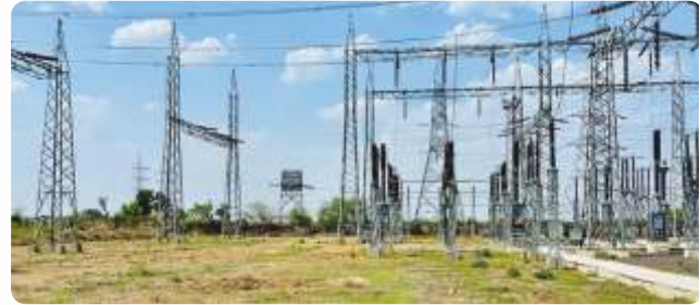
Substation Augmentation at Umred Nagpur, MH | 220kV
